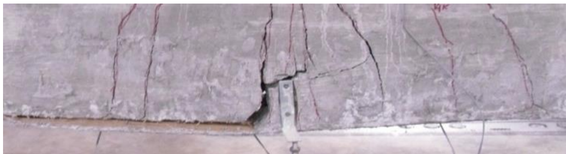
Figure 2. 5 - Debonding failure occurred in a four-ply strengthened beam, Leardini et al. (2013)
