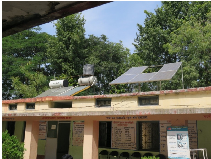
Fig. 2.2: Solar PV system and solar collectors installed on the roof of Katgaon hospital
