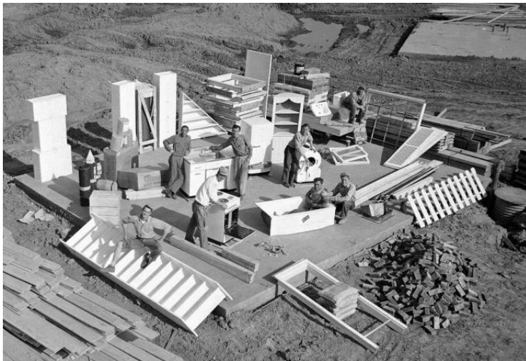
Levittown , all the pieces needed to compose a house are delivered on site and built within 3-4 days.
