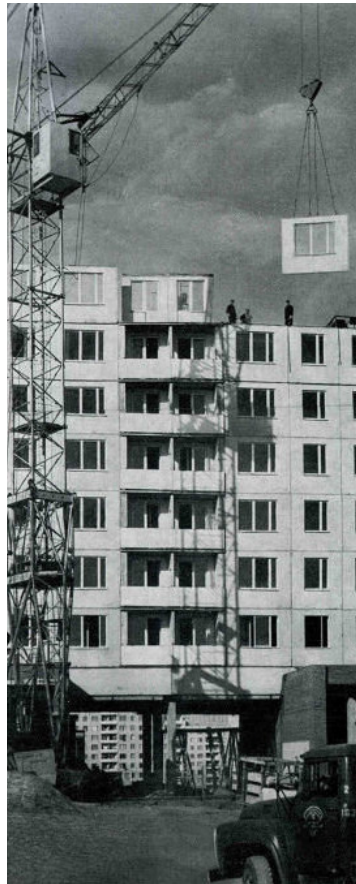
Khrushchyovka, frame of a documentary showing the contracting system with the help of a crane.
