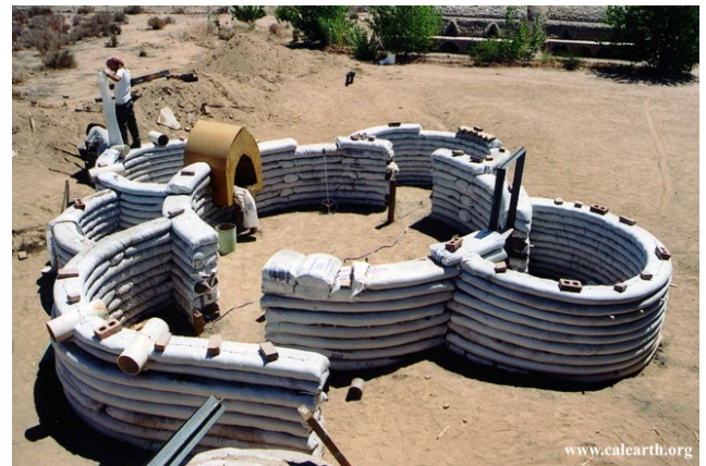
Figure 2.24 : Construction of the Eco Dome. For each room a string is staked to ground in the at the center of curvature, the string is then used as a guide as the structure is built up so that each layer is evenly distributed. Image source: www.calearth.org
