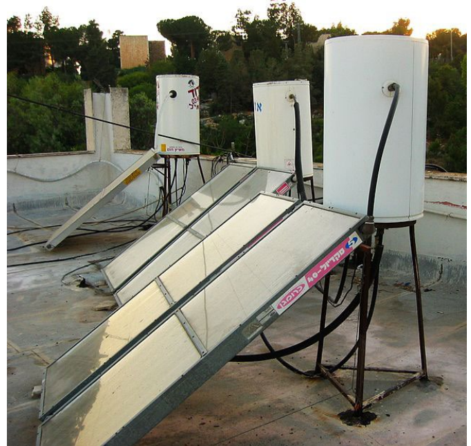
Figure 2.35 : Passive (thermosiphon) solar water heaters on a rooftop in Jerusalem, Israel. [67]
