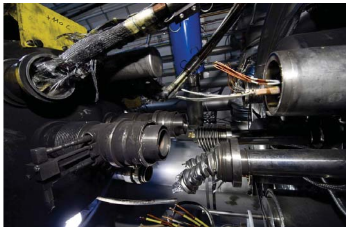
Figure 4.1: Visible damage to the LHC magnets in sector 3-4 of the LHC on November 12th, 2008. On September 19th, 2008, as the LHC was being switched on, a faulty electrical connection between two of the accelerator's magnets caused a large helium leak, which violently vented 6 tons of helium into the tunnel. The resulting temperature rise damaged some 53 magnets (courtesy of CERN).
