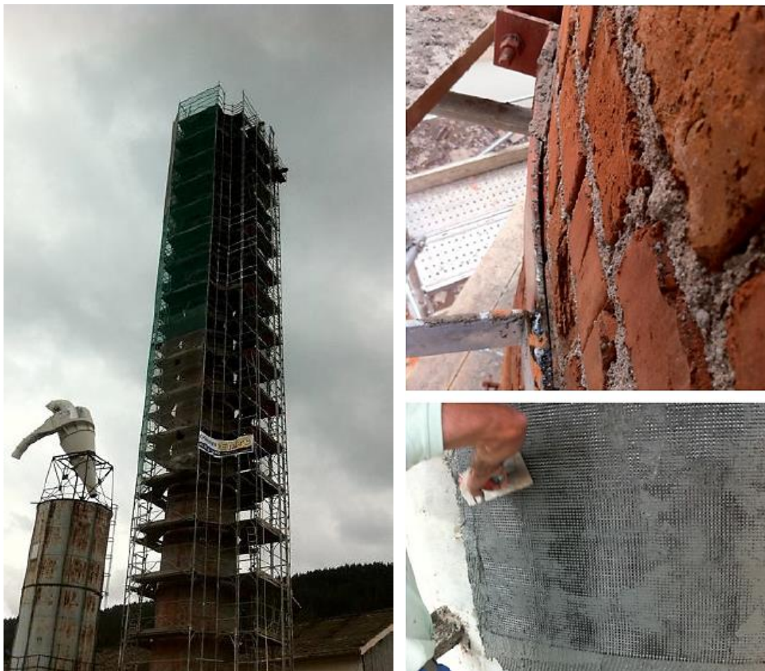
Figure 2.10 – Left: Chimney surrounded by scaffolding during repair. Right: Chimney masonry surface before and during strengthening (Nanni 2012)
