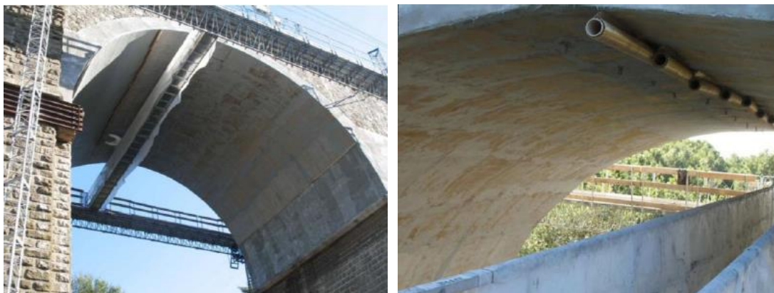
Figure 2.7 – Left: Workers install the first layer of PBO-FRCM on the soffit of concrete vault. Right: Application of the second ply of PBO fabric (Nanni 2012)
