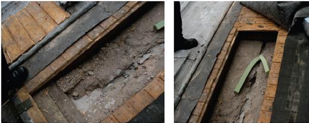
Figure 2.8 – Photograph of the crack through the roof above the octagon (Buttner et al. 2011)
