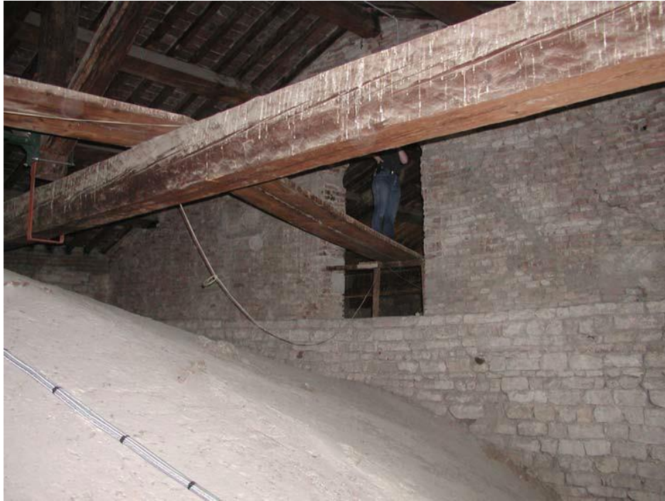
Figure 10 Cracks and repaired cracks on the transverse wall between Bays 3 and 4
