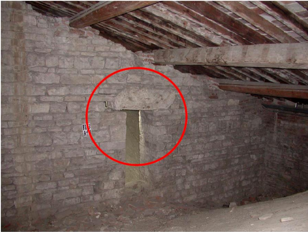
Figure 11 West Aisle: transverse wall between Bays 3 and 4. Cracking and shifting of the stonework of up to 20 cm has been noted
