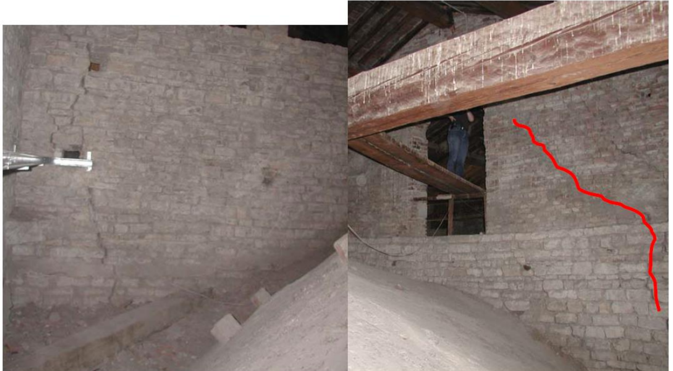
Figure 16 Crack patterns suggestive of influence of wall ties on transverse nave walls
