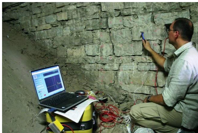
Figure 23 Carrying out a sonic test on the transversal walls of the Basilica of St. Maria Novella
