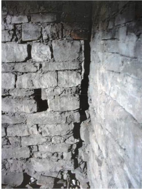
Figure 15 Junction between transverse aisle wall between Bays 3 and 4 and west wall of church
