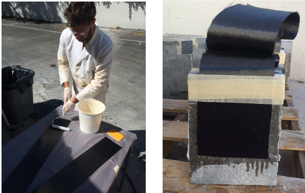
Fig. 2. 42- Impregnation of the FRP sheet (left) and specimen after the installation of the FRP sheet (right)
