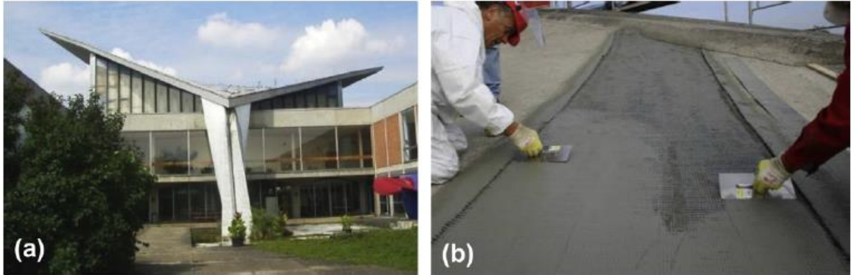
Figure 3.16: (a) Damage hyper-shell at the FH Schweinfurt (Germany), (b) strengthening with TRC process [Mechtcherine 2011].
