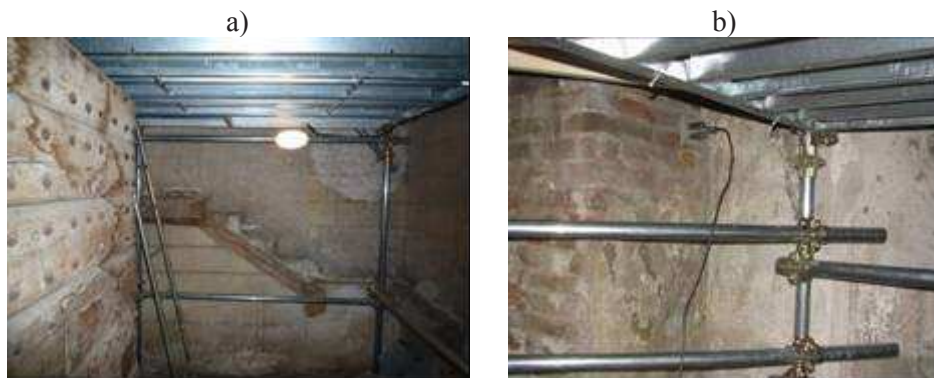
Figure 4.18 View of the metallic scaffolding installed after Summer 2012 (a) and typical inner mounting of the accelerometers in the second AVT (b)
