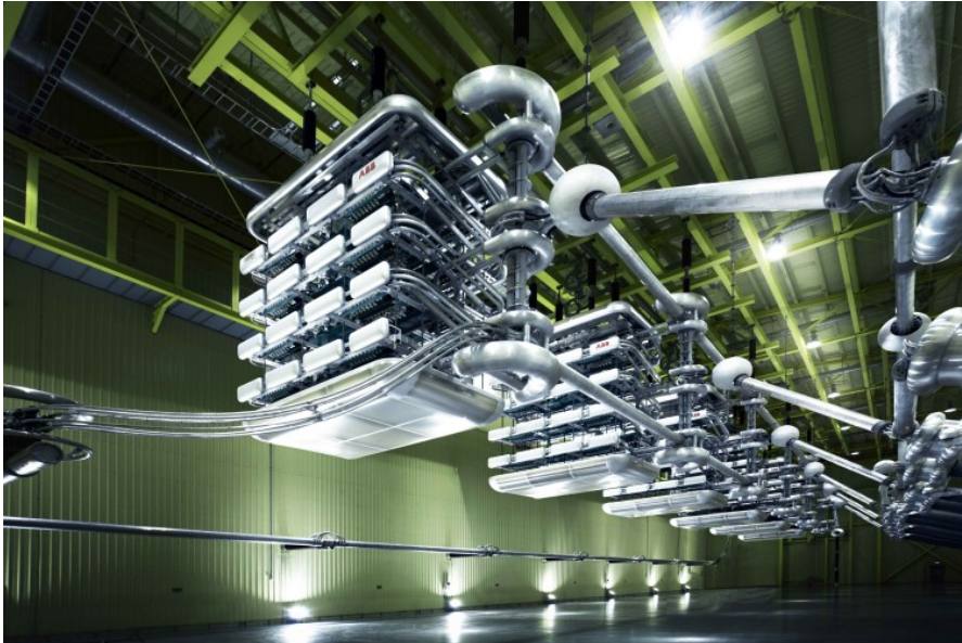
Figure 1.1.: An array of thyristor valves in an ABB HVDC converter station. (image from [12])
