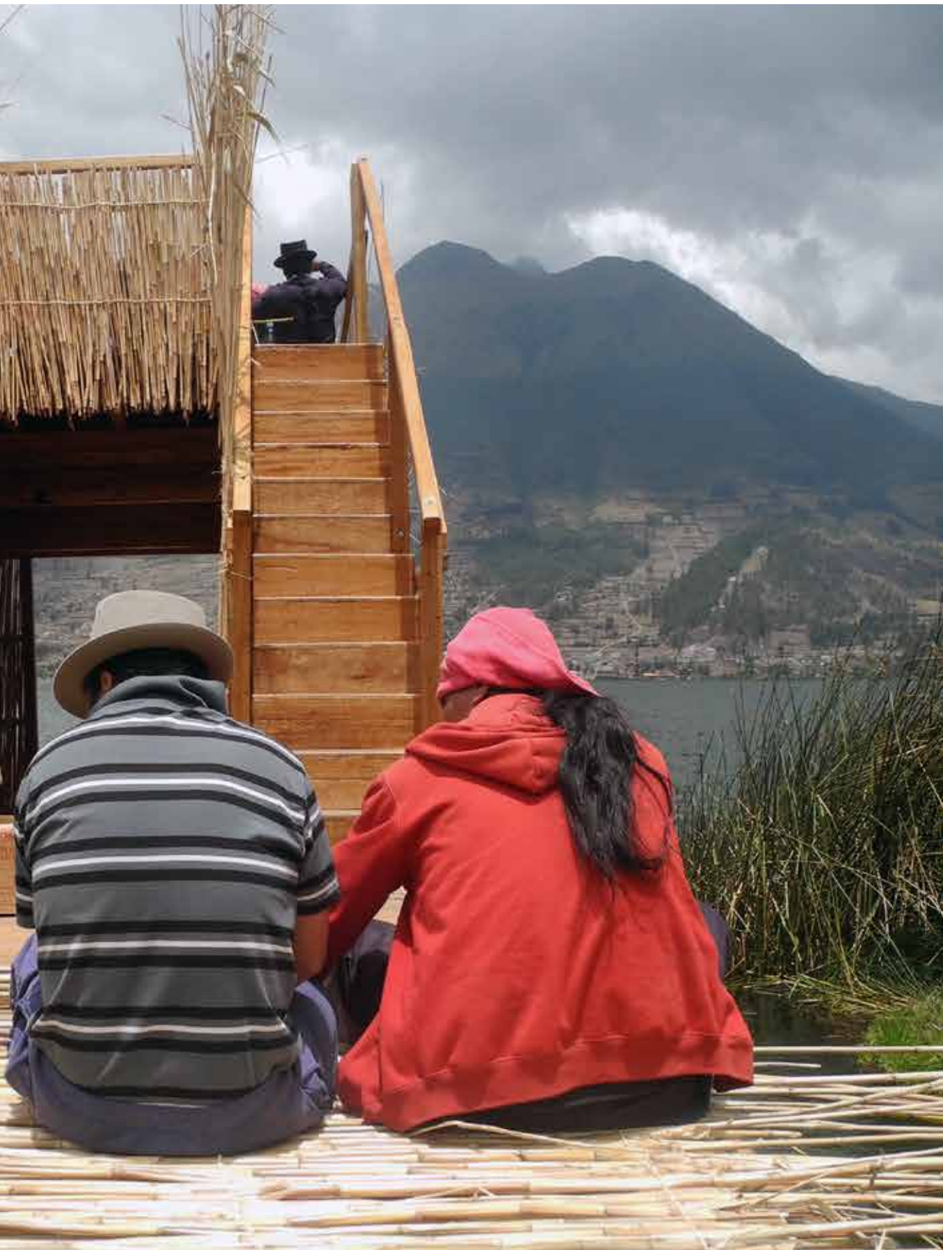
Photo: Construction site situation - week 6: Francisca, Jose and Jaime interlacing carrizo, Cachiviru.
