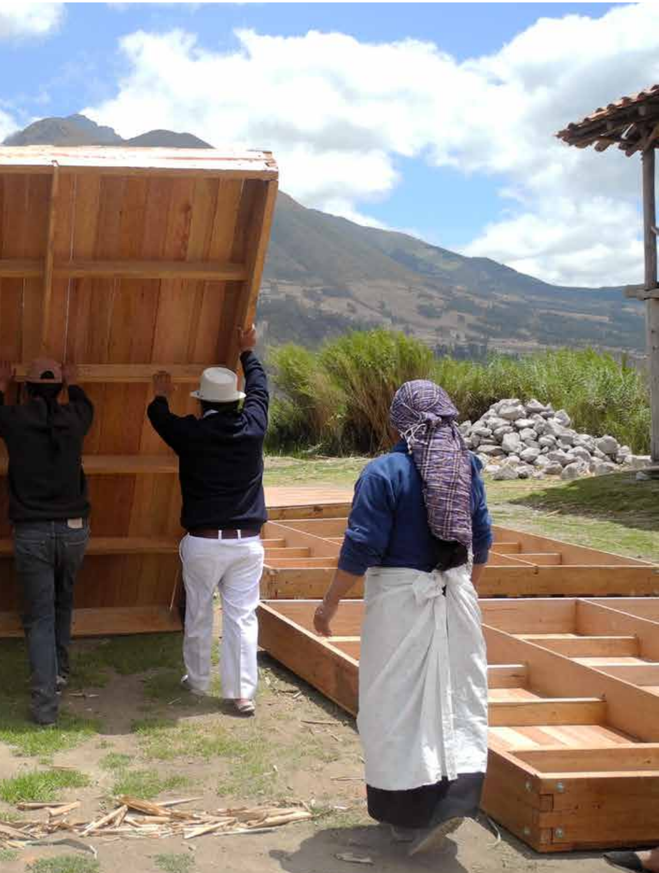
Photo: Community turning over floating modules to put the tanks, construction site, Cachiviru.
