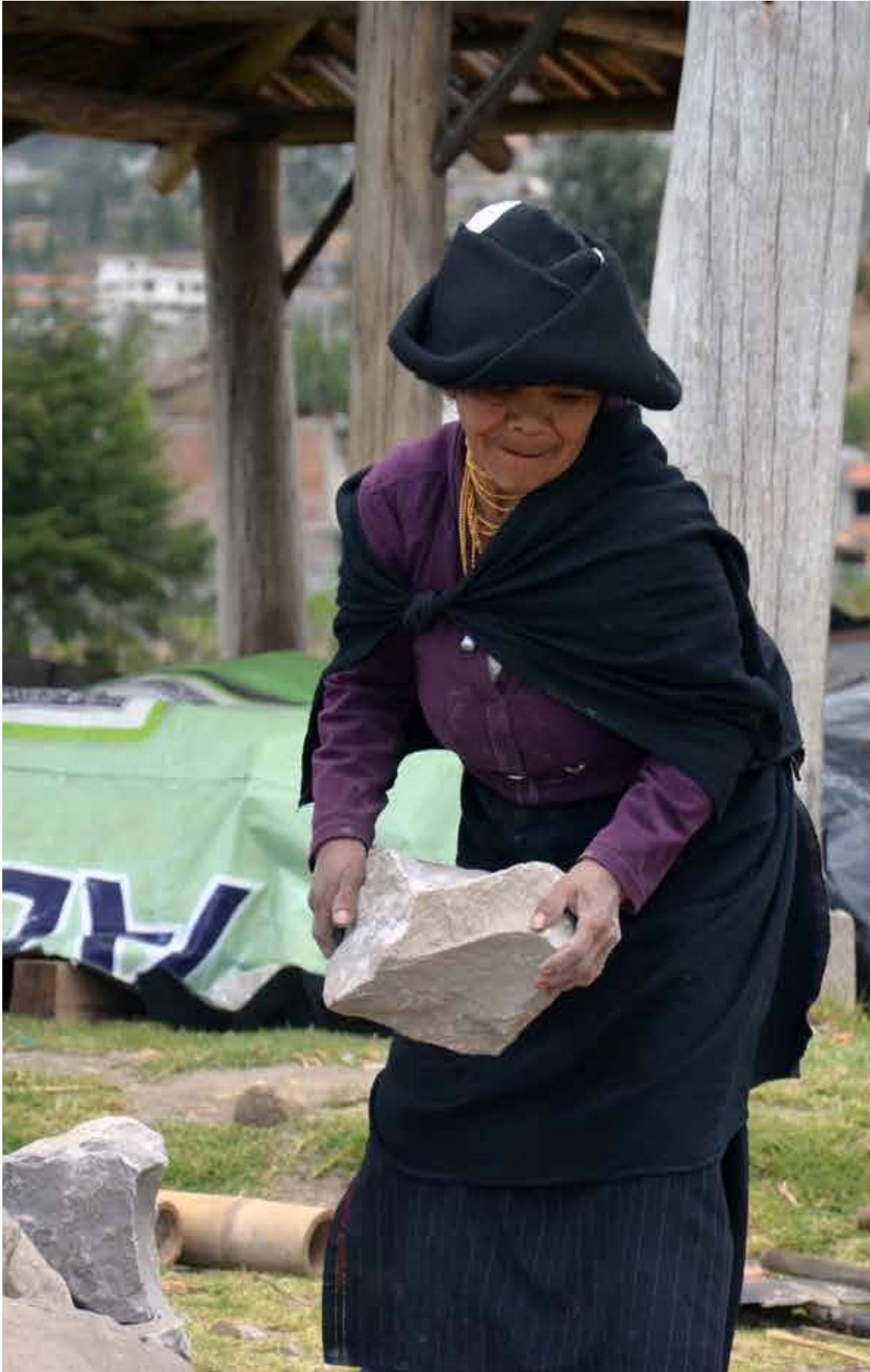
Photo: Maria transporting a big stone to be put into the gabion, construction site, Cachiviru.
