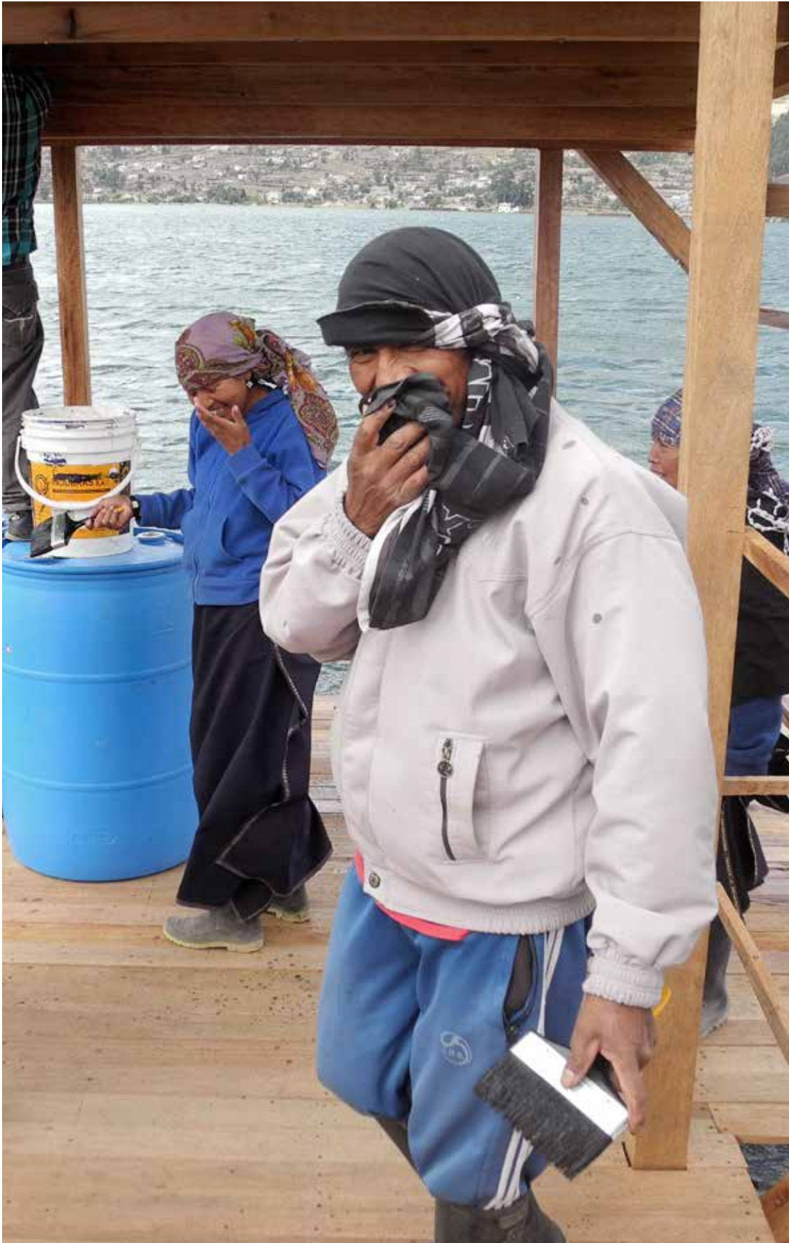
Photo: Mirador varnishing work in progress (Patricio not really happy about the smell!), construction site, Cachiviru.
