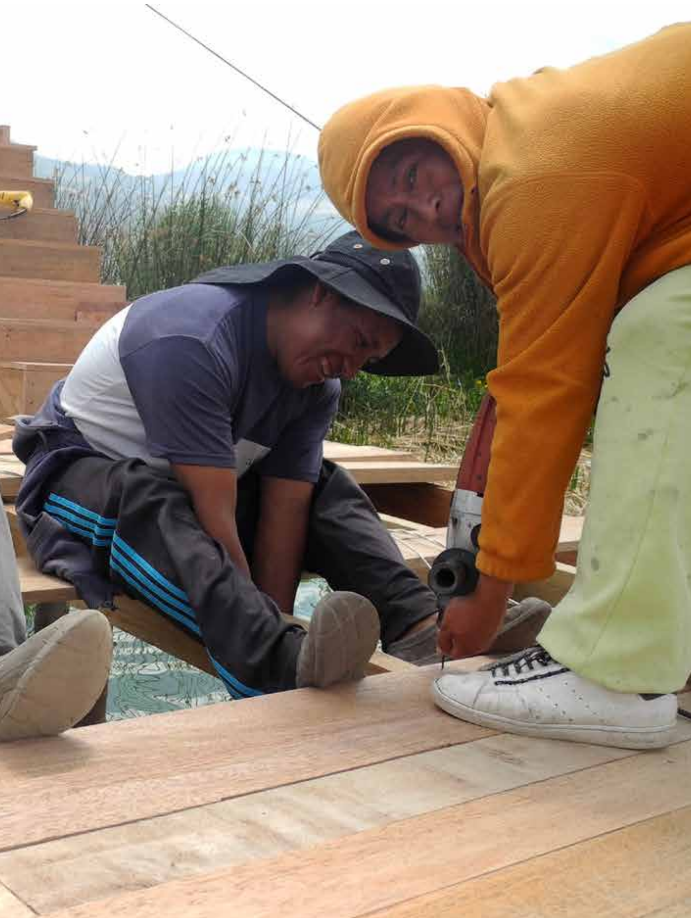
Photo: Jaime, Jose and Gregorio bolting the flooring to the boardwalk structure, construction site, Cachiviru.
