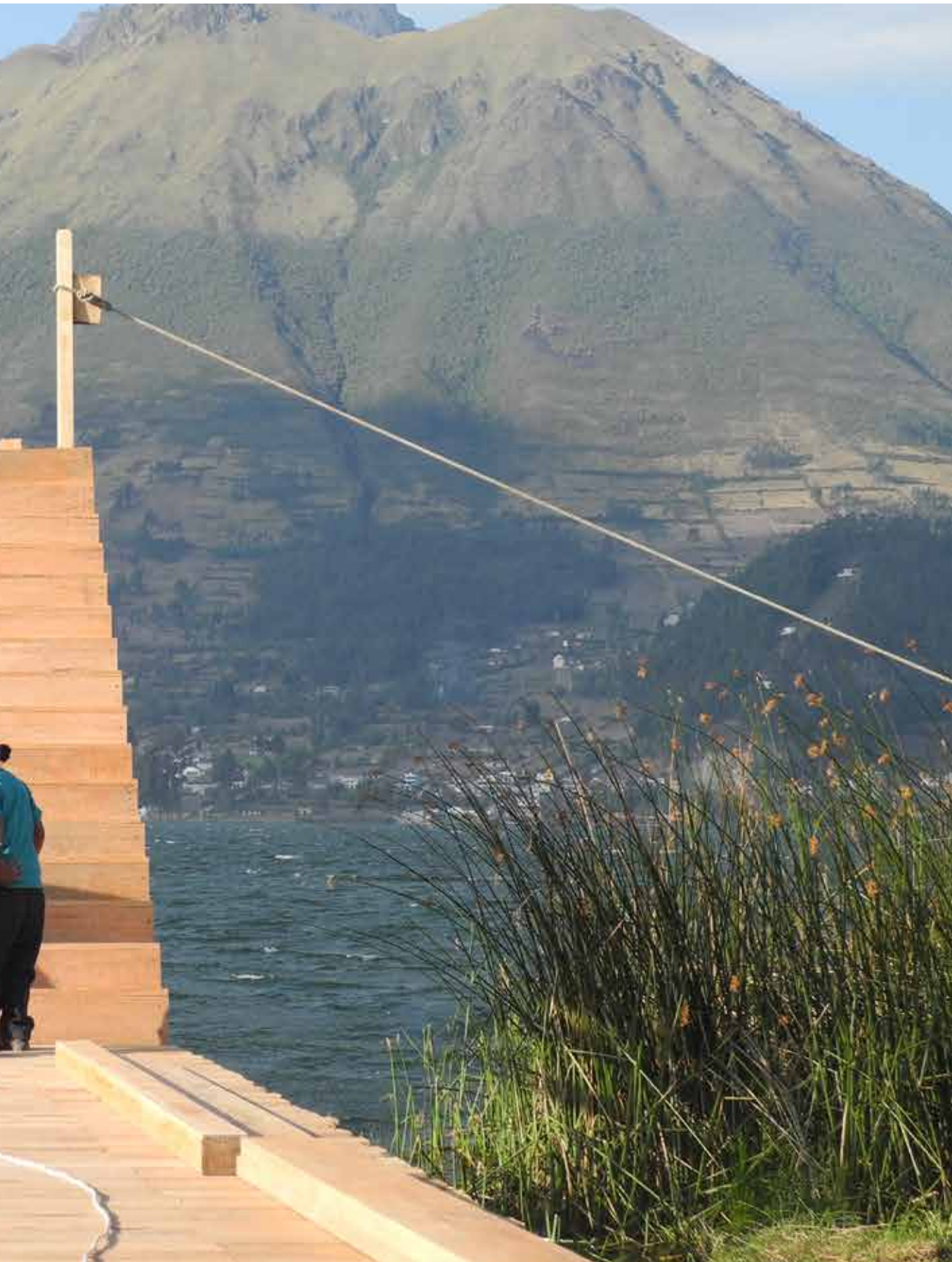
Photo: Construction site situation - week 3: children enjoying the view while "Negro" is working, Cachiviru.
