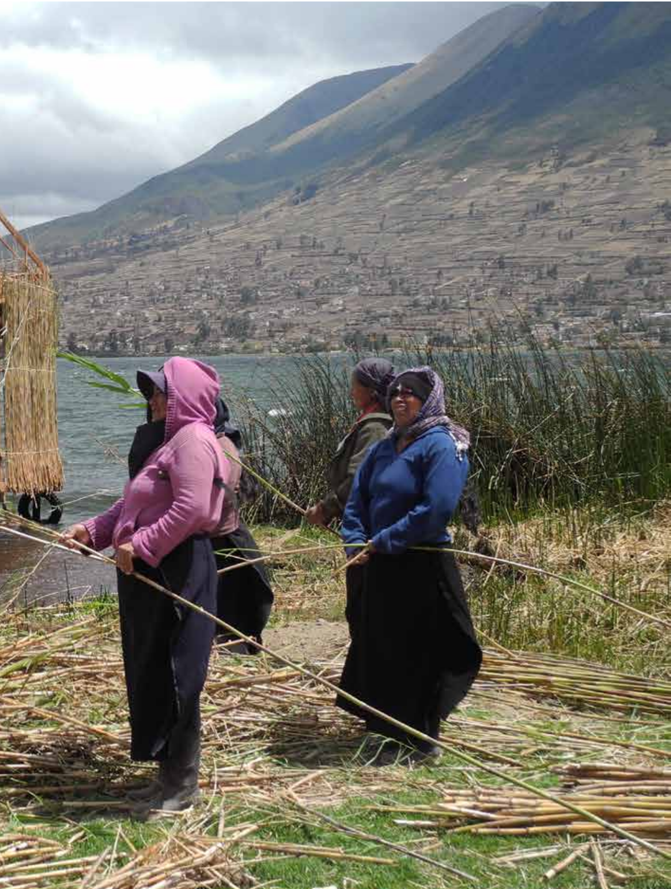
Photo: Construction site situation - week 7: community preparing the last carrizo to be put on Mirador, Cachiviru.
