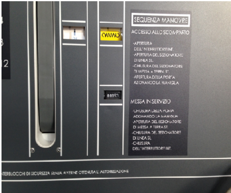
Figure 4.7: Counter of the number of times the circuit breaker has worked
