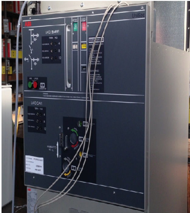
Figure 4.6: ABB Switchgear, the cabinet where the Thyssensor and ABB circuit breaker houses
