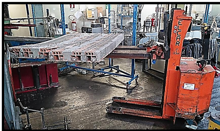
Figure 27. Lift truck to place the slab in the correct position. (Source: Laboratory image)
