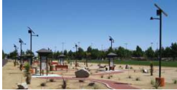
Figure 1-26: Pathway and Trail Lighting
