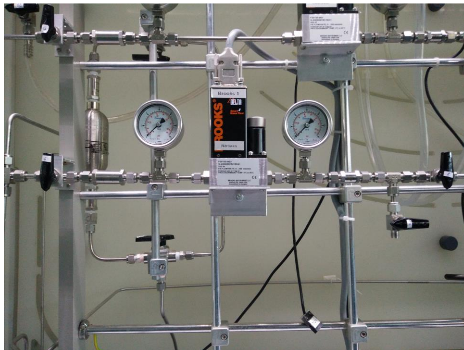
Figure 3.2: Flow control equipment ( Mix AC2 line )
