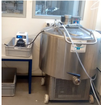
Figure 3-3 Milk tank used for the storage of the incoming wastewater
