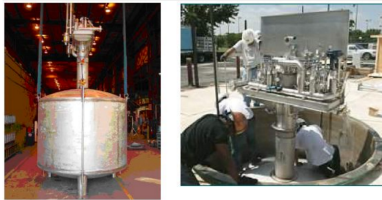
Figure 1.11: Air Products' underground LH_2 tank being installed at the Shell Hydrogen refuelling station in Washington DC in 2004.
