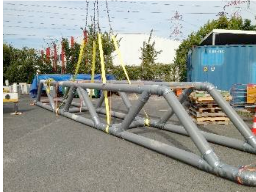
Figure 2.20: The structure is moved to its definitive support once concrete has hardened.
