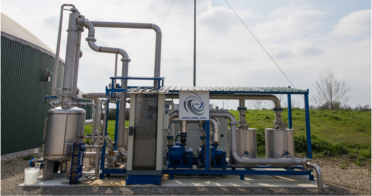
Figure 5-16: The pre-treatment unit for biogas in CAT biogas plant in Correggio (RE).
