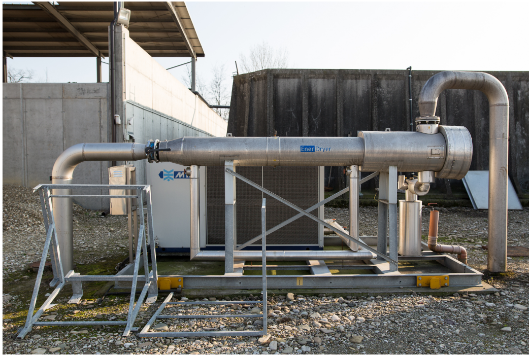
Figure 5-10: Chiller pretreats biogas before approaching engines in order to decrease H 2 O content
