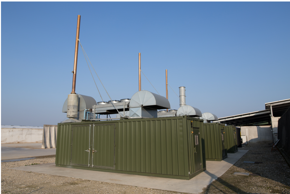
Figure 5-9: Three 333kW MAN engines inside containers explosion proof
