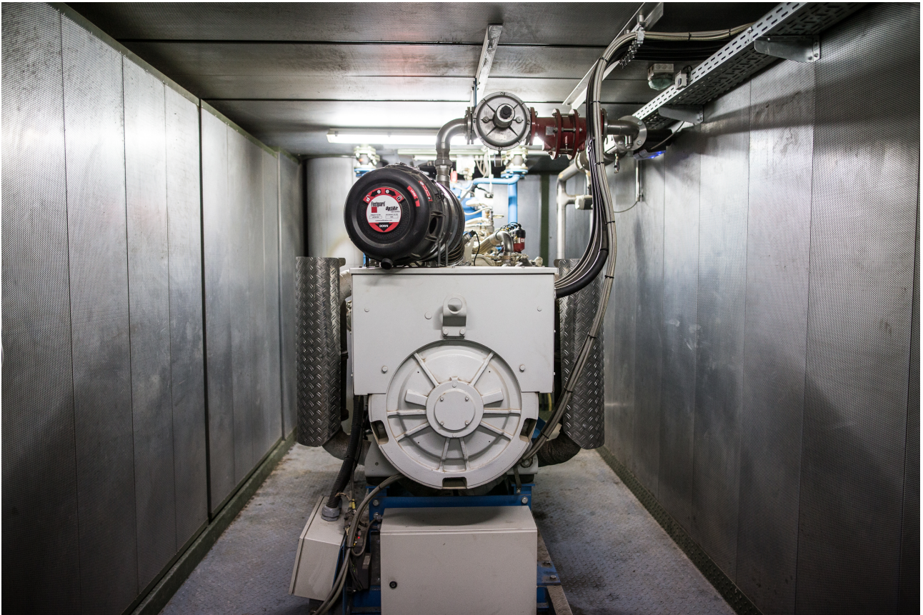
Figure 5-8: A view of Engine MAN 333 kW in “Valtrebbia Energia” Biogas Plant
