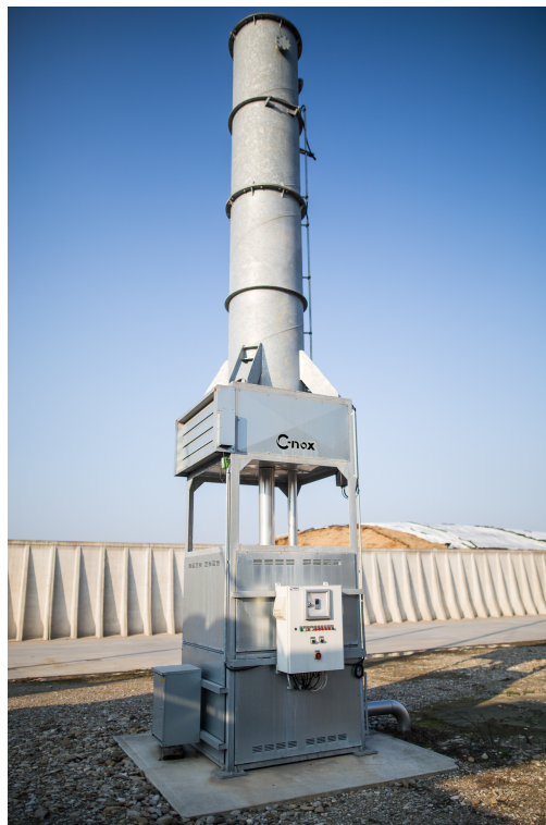
Figure 5-6: Flare located into “Valtrebbia Energia” Biogas Plant. On background substrate storage tank can be appreciated.
