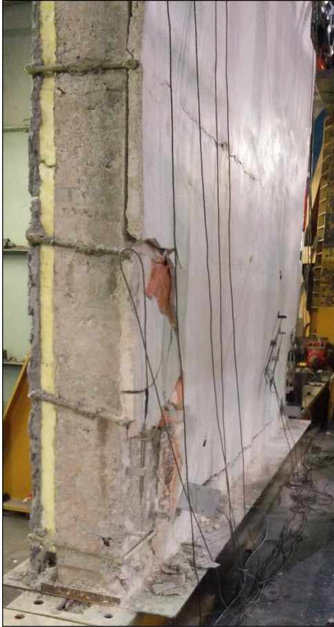
Figure 5-6. Fifth cycle damages
