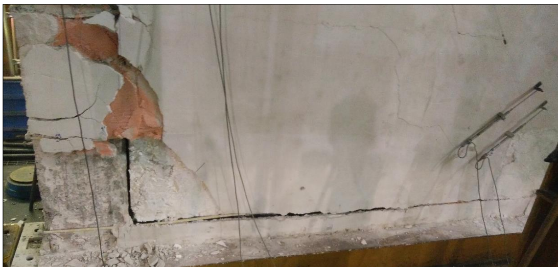
Figure 5-10. Infill separation from the frame
