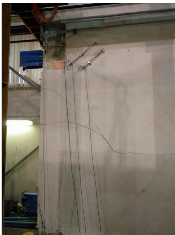
Figure 5-1. First cracks in the mortar
