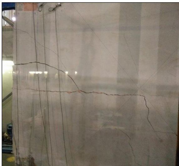
Figure 5-2. Growth of the old and creation of the new cracks
