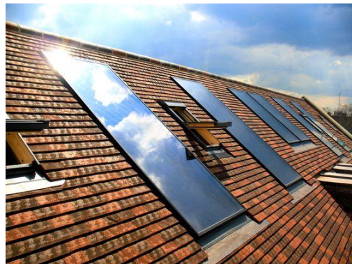
Figure 37 – Integrated Solar Thermal Collectors [source: http://www.viridiansolar.co.uk/ ]
