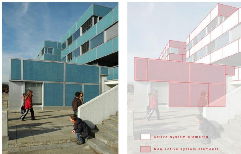
Figure 7 – Solar thermal façade elements (dark blue and red) and dummy elements (light blue and white) [18]
