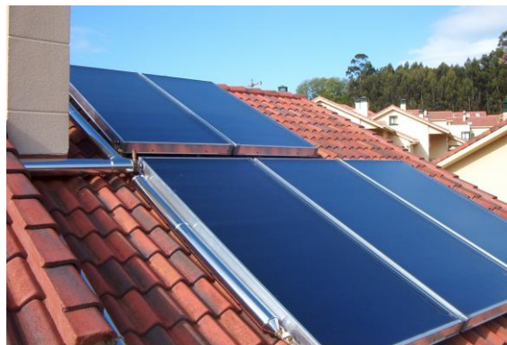
Figure 36 – Partial Integrated Solar Thermal Collectors [source: http://www.genera.pt/energias/energias-renovaveis/ ]
