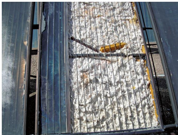
Figure 41 - Corrosion of a STC's components after the glass cover is broken [77]
