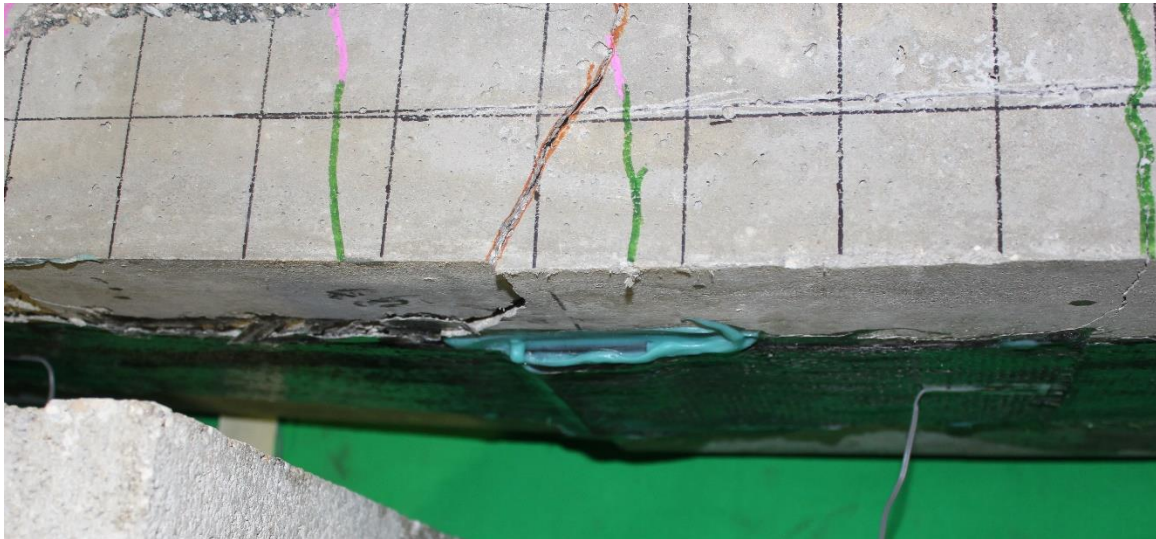
Figure 6.42 - Slab 003 failure details
