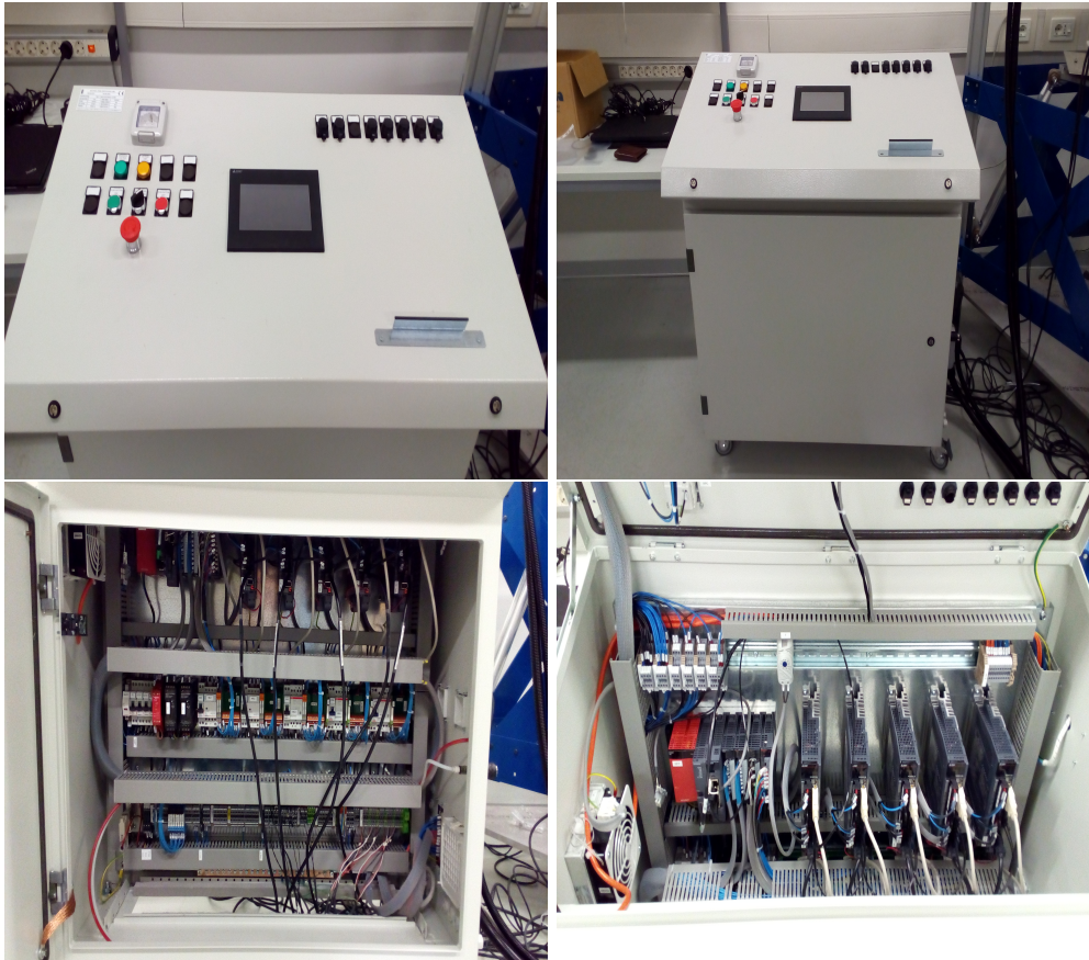
Figure 3.5: final result of the electric cabinet
