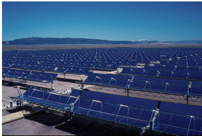
Figure 1.6 SEGS Parabolic Through, California, taken from [9]
