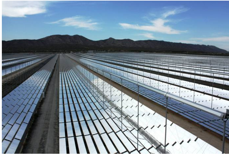
Figure 2.2: Linear Fresnel Reflector installed at PE-2 plant [23]
