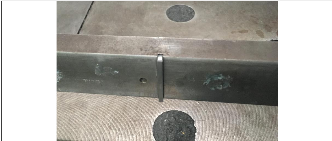
Fig. 3-57 Crack in the beam
