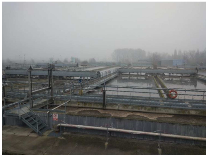
Figure 12. Actual sedimentation tanks with traveling bridge.
