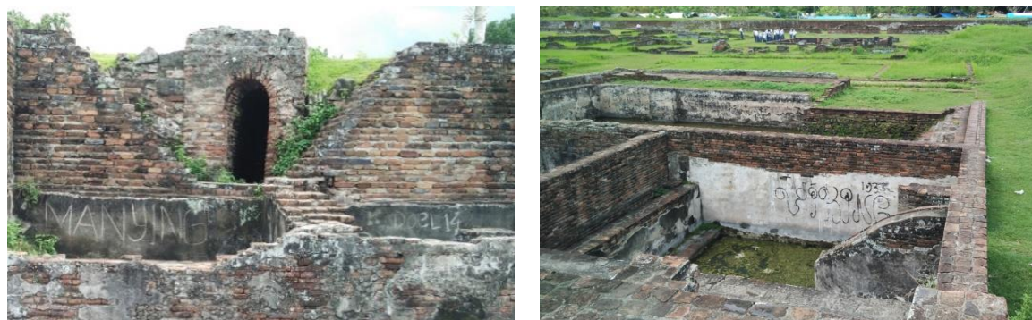
Figure 60. Vandalism that happens around the relics.
