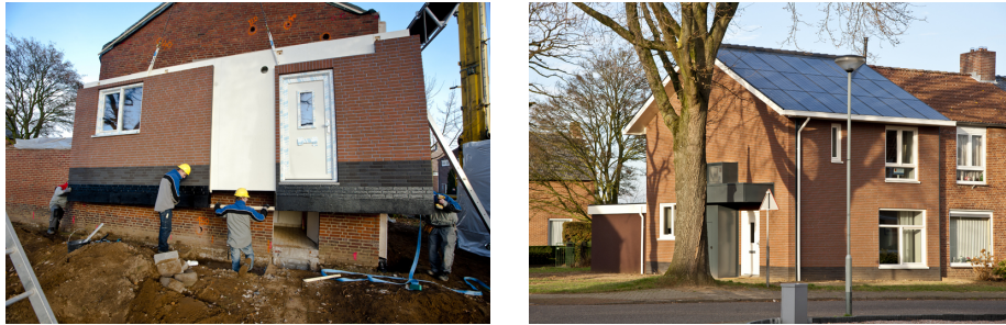
Figure 3.5: Stroomversnelling - Implementation of prefabricated facade modules and final result after renovation. (Rovers, 2014)
