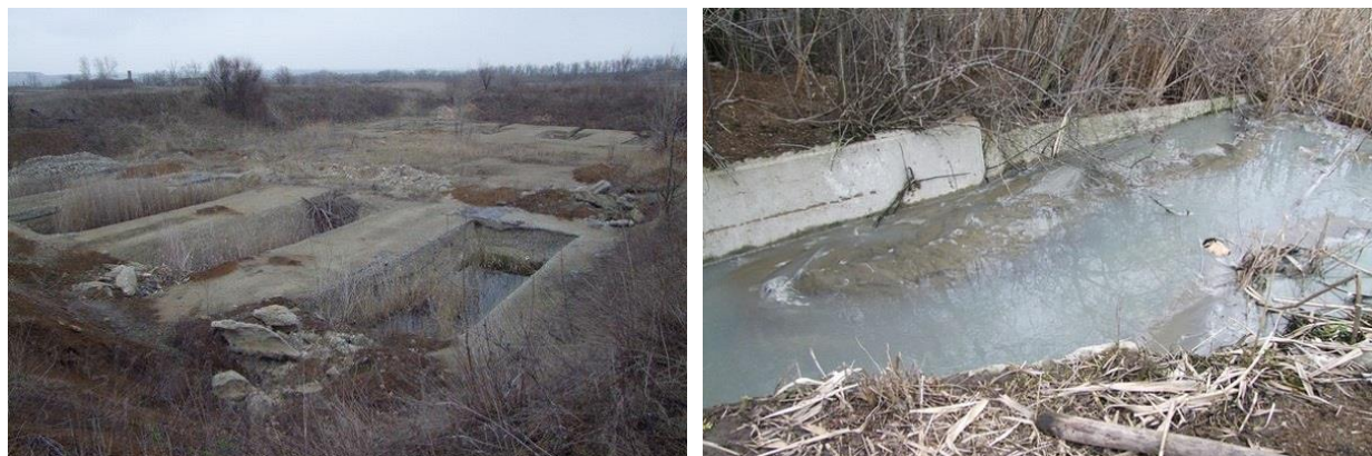
Image 4.5.15. The conditions of wastewater treatment plant in Zverevo in 2016.
