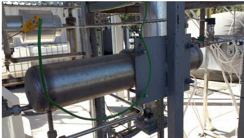
Figure 2. 10 - Inlet absorption column gases cooler
