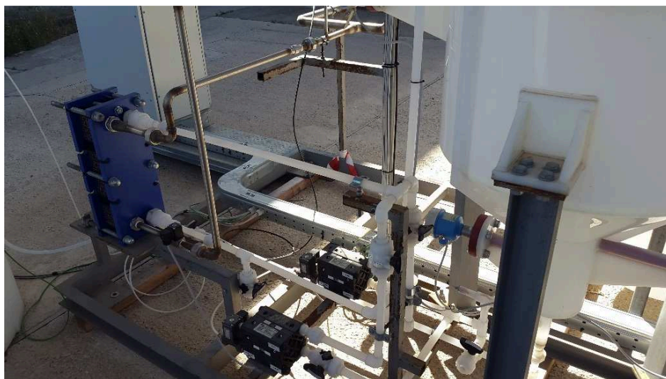
Figure 2. 12 - Plate heat exchanger and recirculating liquid pumps detail
