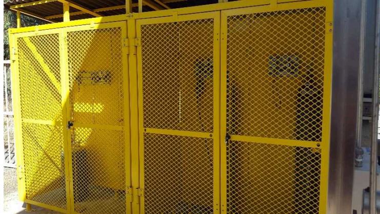
Figure 2. 5 - Safety box and storage area for gas bottles
