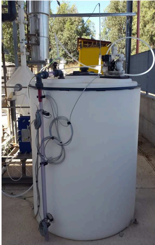
Figure 2. 13 - Storage tank for commercial grade H 2 SO 4
