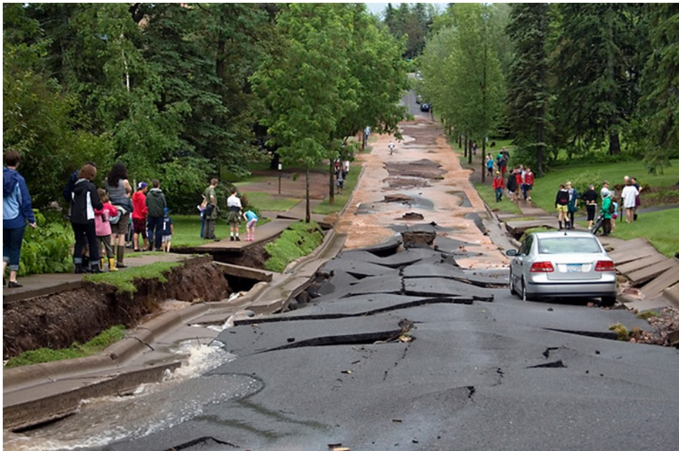
Figure 2.7: Heavy damage to a road in Duluth, Minnesota June 2014
