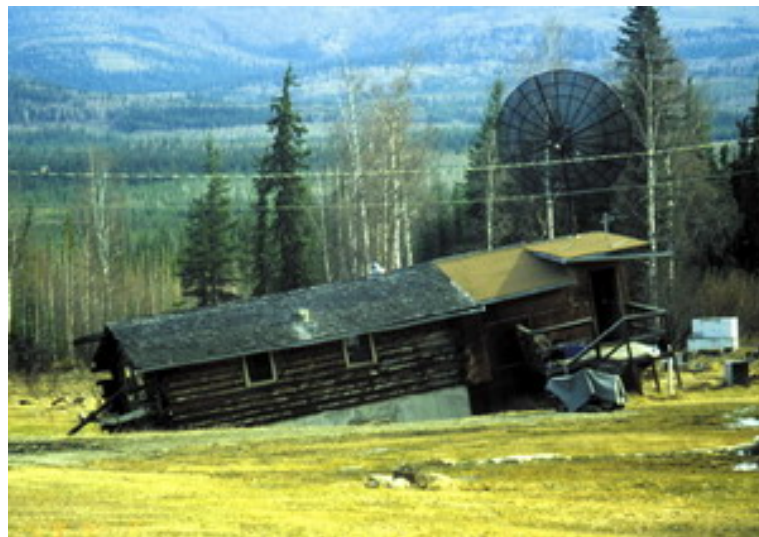
Figure 2.3: Sinking house. Effects of non-thaw stable permafrost on heated foundations in the hills surrounding Fairbanks
