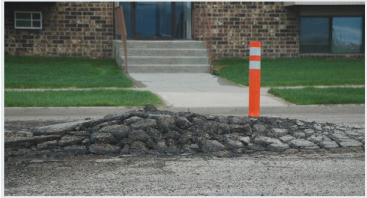
Figure 2.6: Frost heave on this Bismarck street has lifted parts of the road surface about 46cm.
