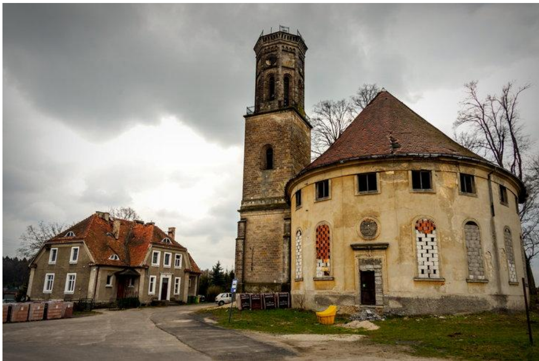
Figure 8. Abandoned Evangelical church in Żeliszów
