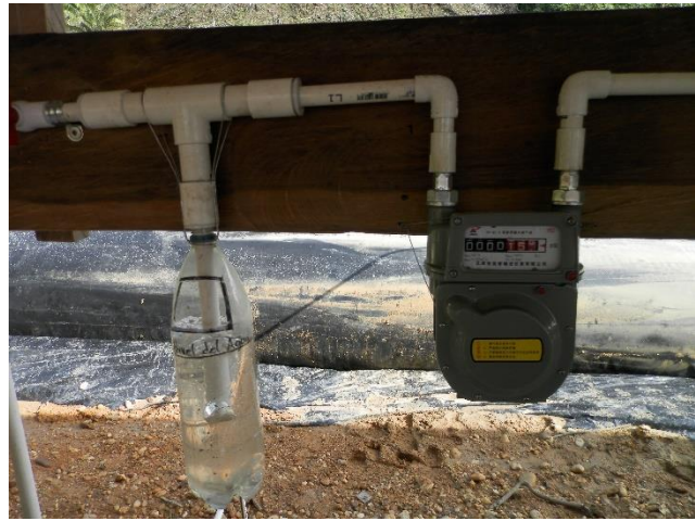
Figure 5.15 Safety valve applied on the line during a working test.
