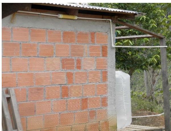
Figure 5.18 H 2 S filter applied on the pipeline.
