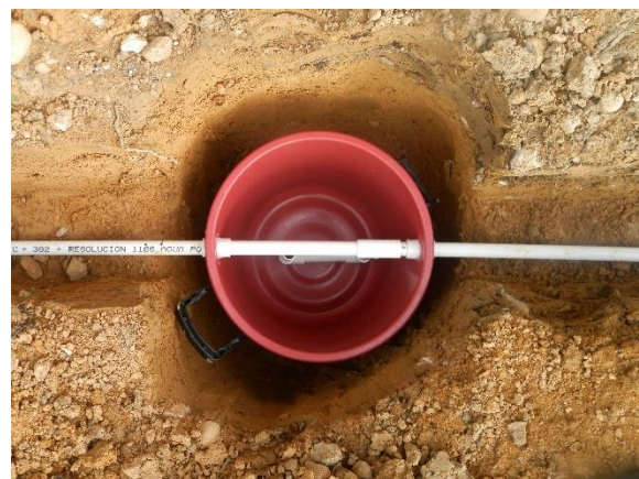
Figure 5.17 Water trap applied on the pipeline.
