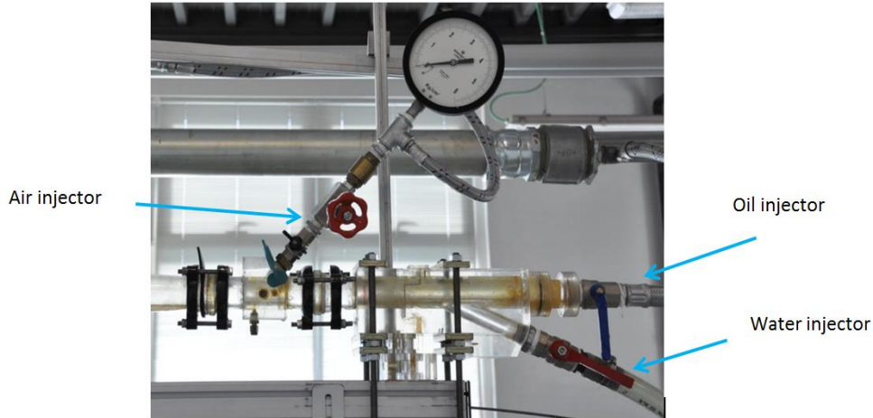
Figure 3-7. Complete view of inlet injector
