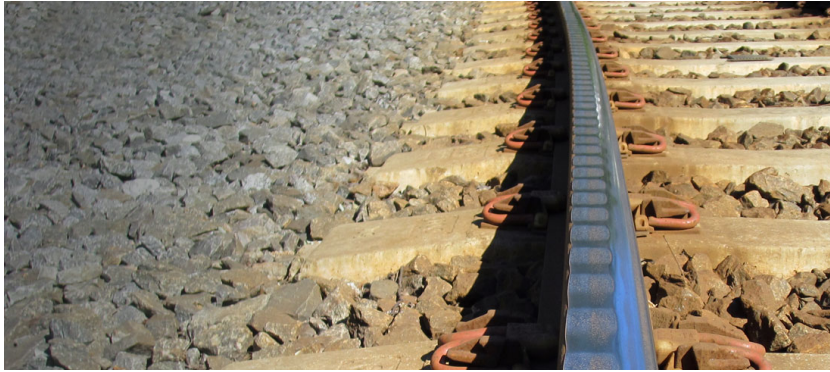
Figure 1.1: Corrugation of the low rail in a tight curve [5]
