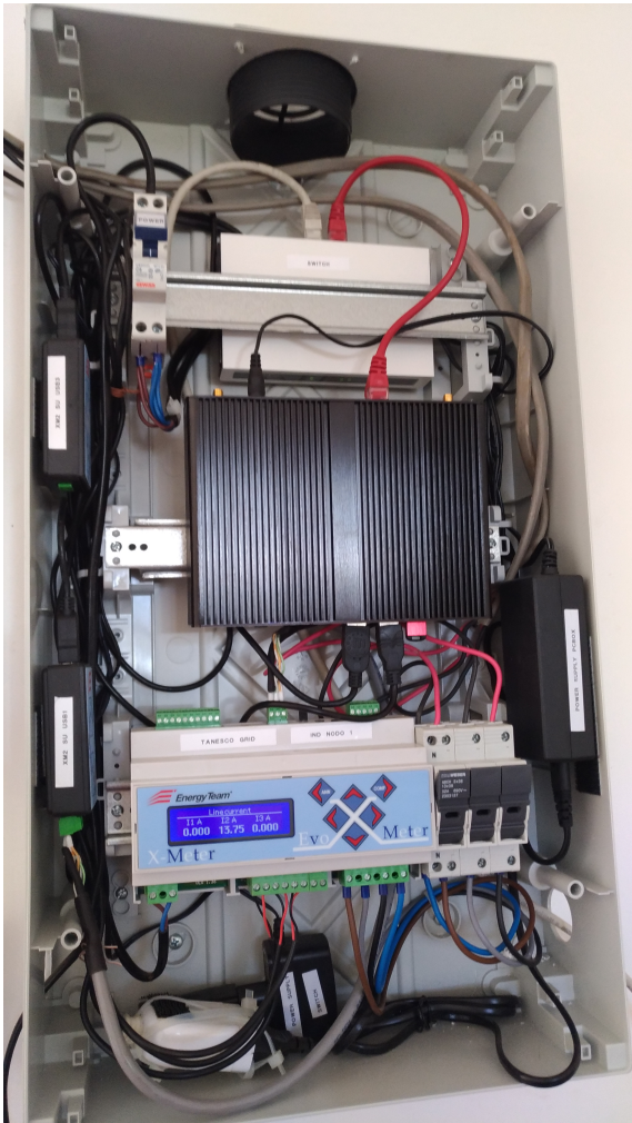
Figure D.3: Picture of the complete electric panel
