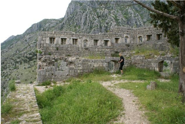
2 Bataglia platform, missing parapet wall and inaccessible walking path
