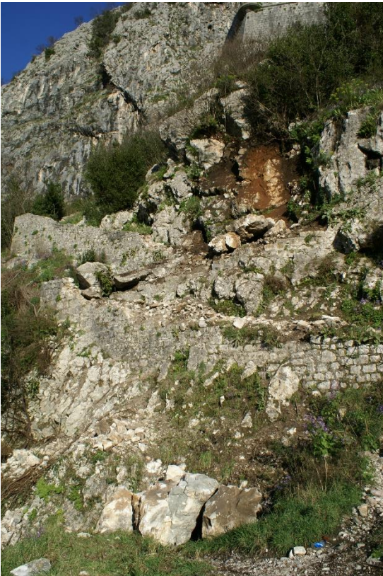
27 Damage caused by landslides
