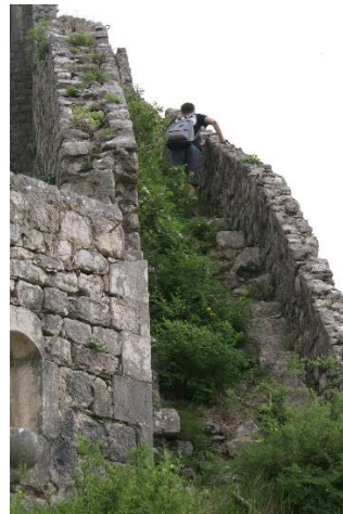
10. Compromised visitors safety
