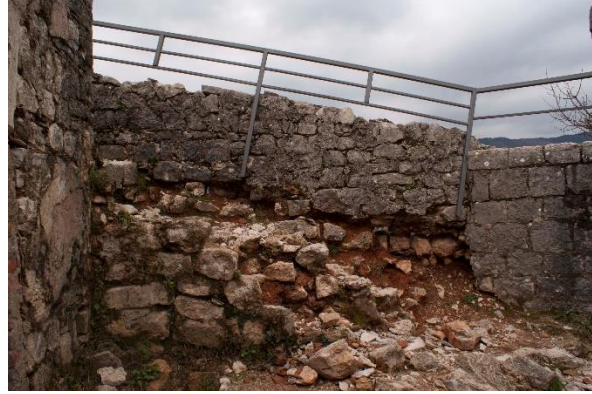
Figure 2. Courtyard wall, decay example
