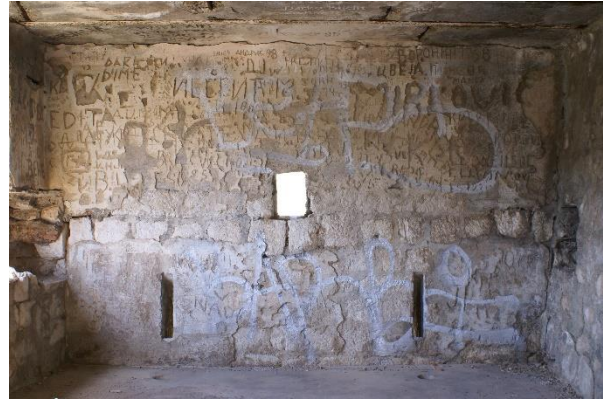
Figure 17. Example of decays
