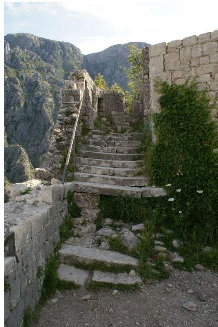
Figure 7. Staircase; example of decay
