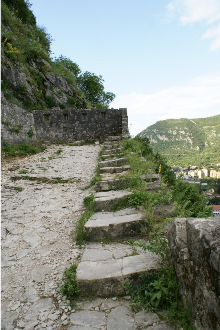
22 Example of missing stone rail
