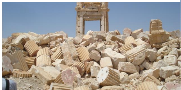
The Temple of Bel after ISIS destruction/ the collapsed pieces, Source: Rania Al-Fahl
