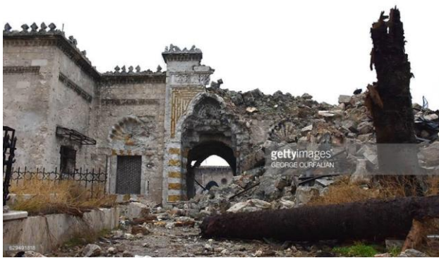
The Northern entrance damaged caused by the destruction of the Minaret, Source: Getty images
