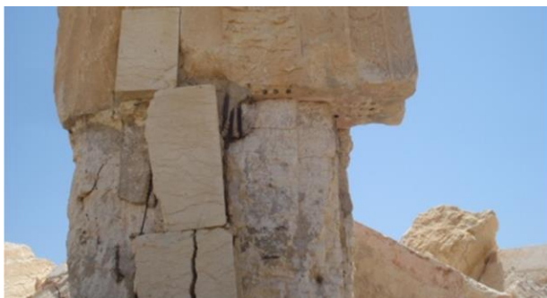
The Temple of Bel after ISIS destruction / The damage of the gate base, Source: Rania Al-Fahl
