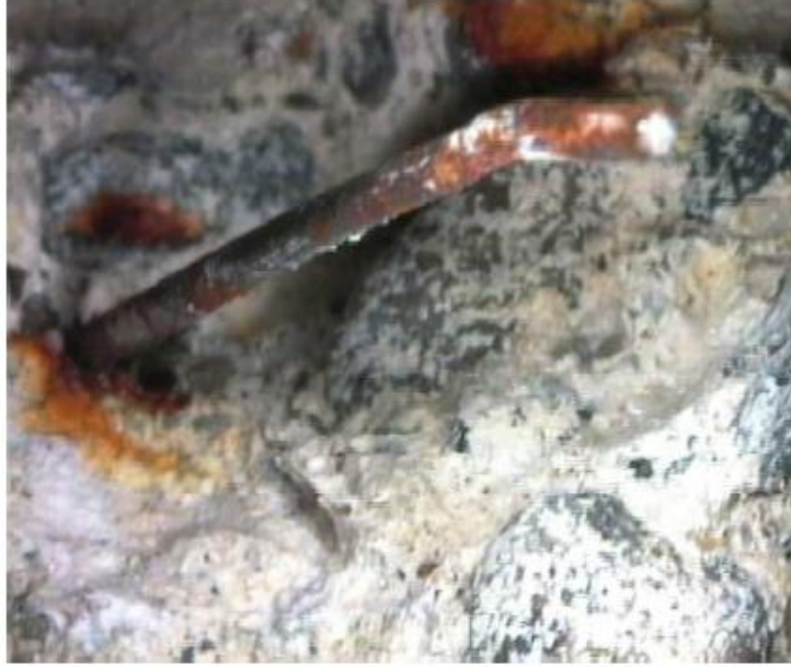
Fig. 2.14 Typical photograph of corroded steel fiber in the crack [288]
