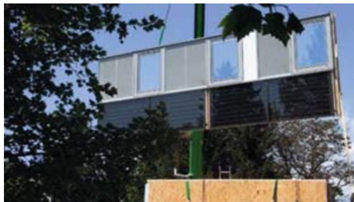
Figure 8 - The solar collectors were integrated into the prefabricated modules.(Source: Gap-Solution GmbH)
