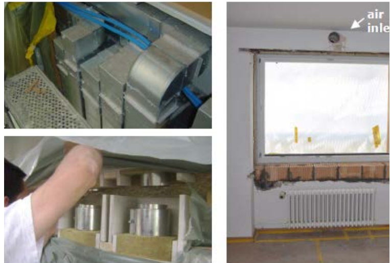
Figure 3 - Ventilation main distribution with space saving rectangular ducts (top left), connecting the telescopic vertical round ducts between façade elements (bottom left), air inlet above window (right)
