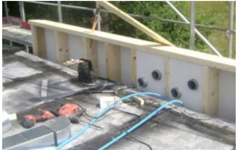
Figure 7 - The step back of the penthouse floor is used for the horizontal ventilation distribution
