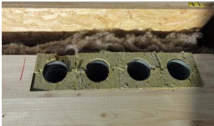
Figure 5 - Mineral fireproof wool protecting the ventilation pipes
