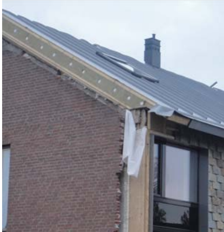
Figure 4 - real section of the timber frame. The external slates and the cellulose insulation are visible, together with the new roof and triple glazing windows
