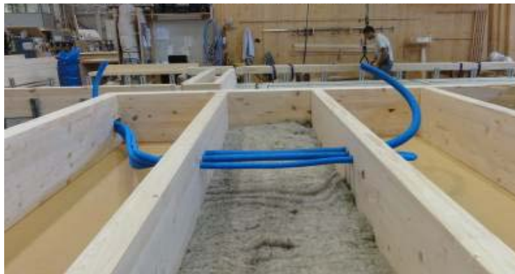
Figure 4 - Cavities for air ducts and electric conduits are integrated into the modules
