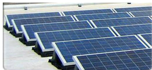
Fig. 5.44 Solar panels on flat roof
