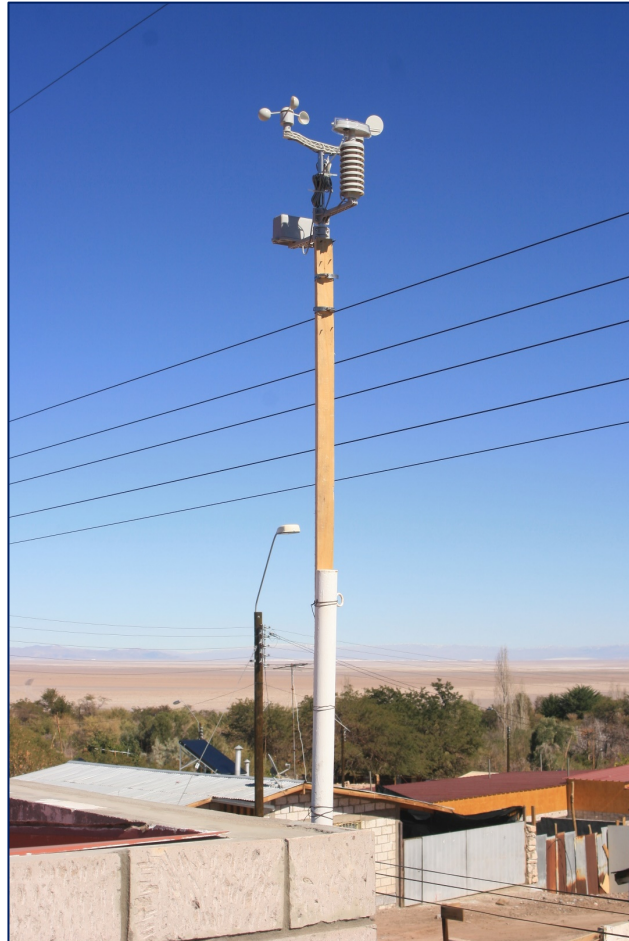
Figure 9: Wind measuring station installed on site. Source: Authors.
