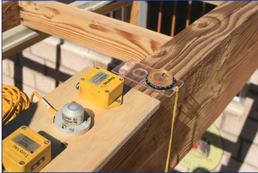
Figure 8: Measuring station installed on site. Source: Authors.
