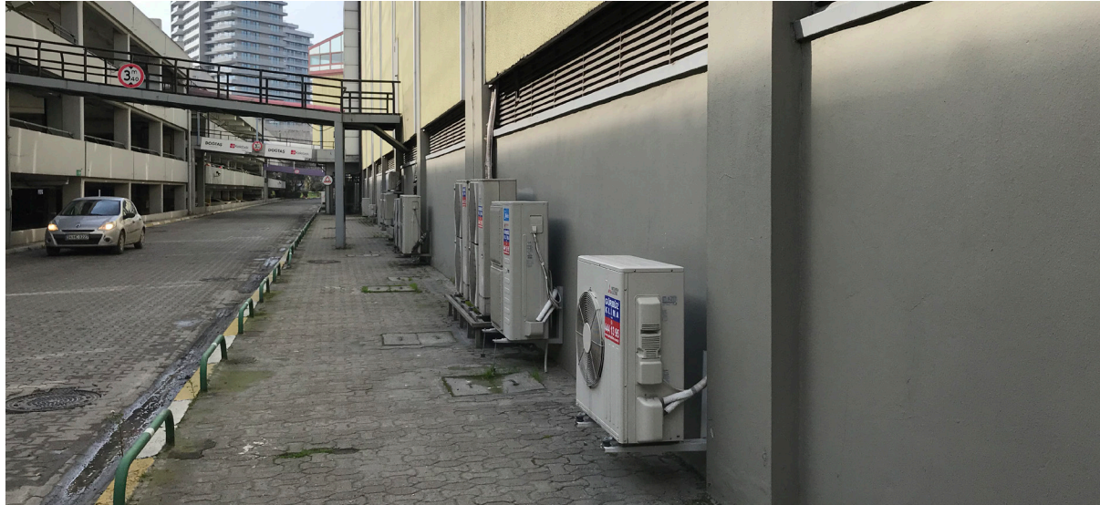
Figure 68. HVAC Systems External Units on the Sidewalk. Source: Author
