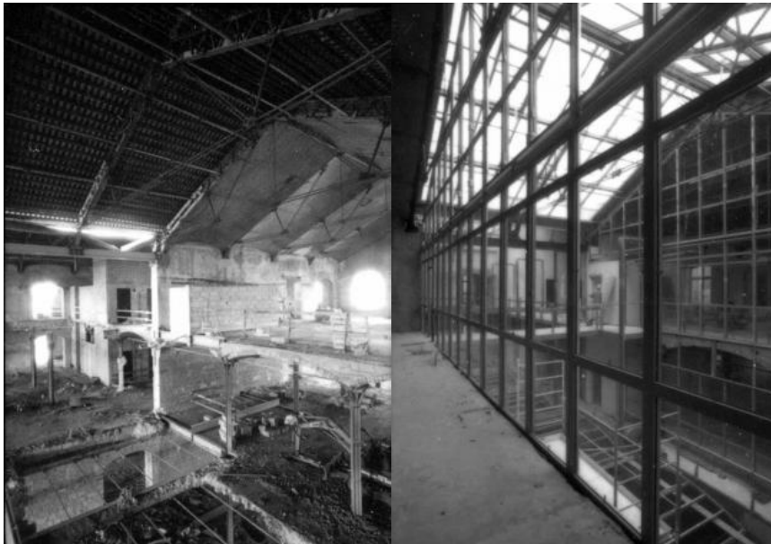
Figure 2.20 Roof replaced by transparent glass roofs to bring natural light inside – Source: Castaldi Archtecte.
