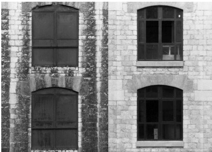
Figure 2.18 The Docks façade. Left: 1991, dirty dark façade, iron binds rusted by sea air. Right: 2001. Façade cleaned up, glass windows respecting the former structure of the iron blinds - Source: Castaldi Architected.
