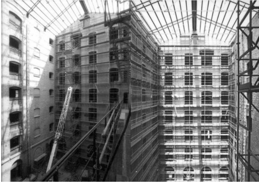
Figure 2.17 Openings enlarged in one of the internal courtyards and roof replaced by transparent glass – Source: Castaldi Architected.
