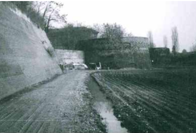
Fig 13: State of the walls before the restoration in 1991
