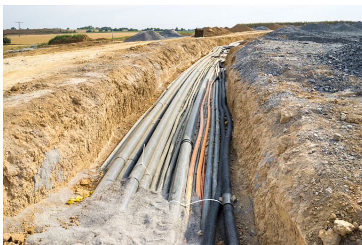
Figure 1-3. Underground high voltage power cables
