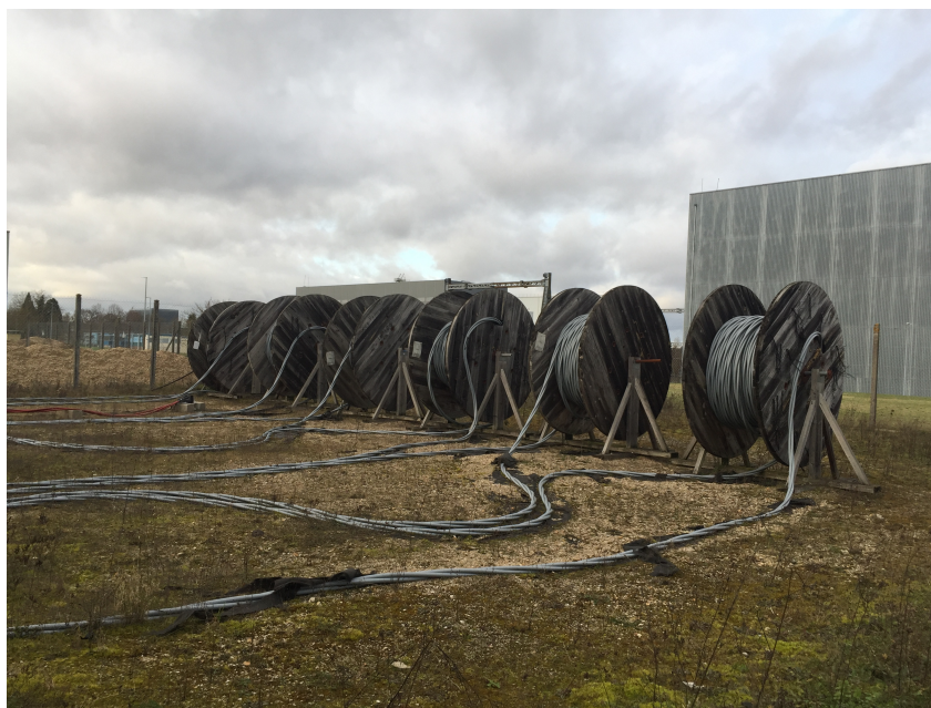
Figure 2-1: Power cables tested in our numerical simulations, EDF Lab Les Renardières, Seine-et-Marne, France
