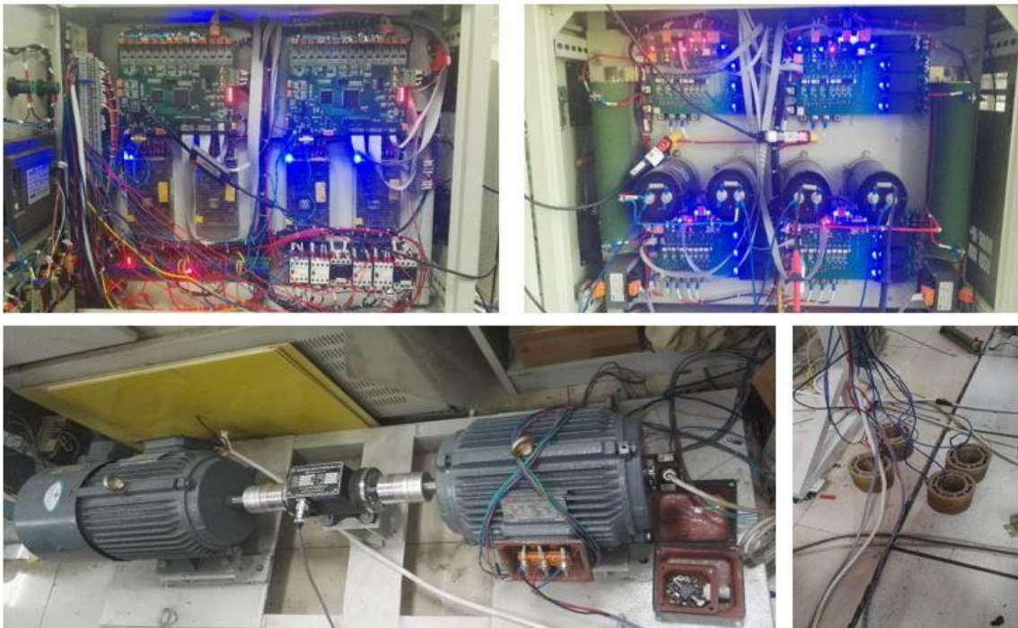
Fig. 4-10 Physical picture of the mutual feedback AC drive test system
