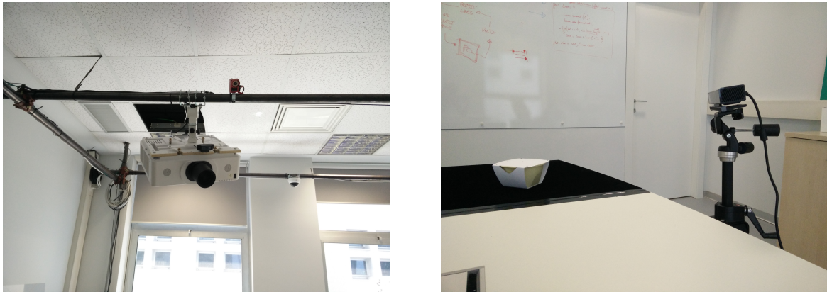
(a) Projector fixed on an upper beam
